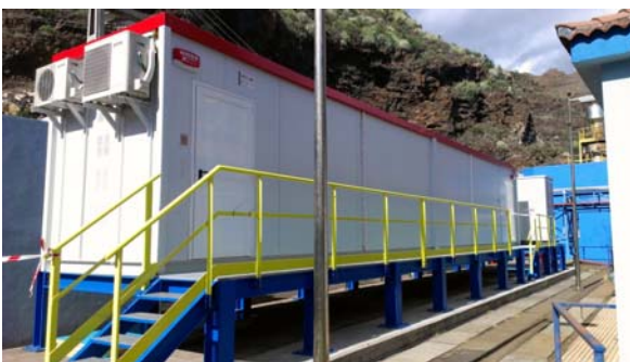
Figure 2: Installation of La Palma ultra-capacitor.
