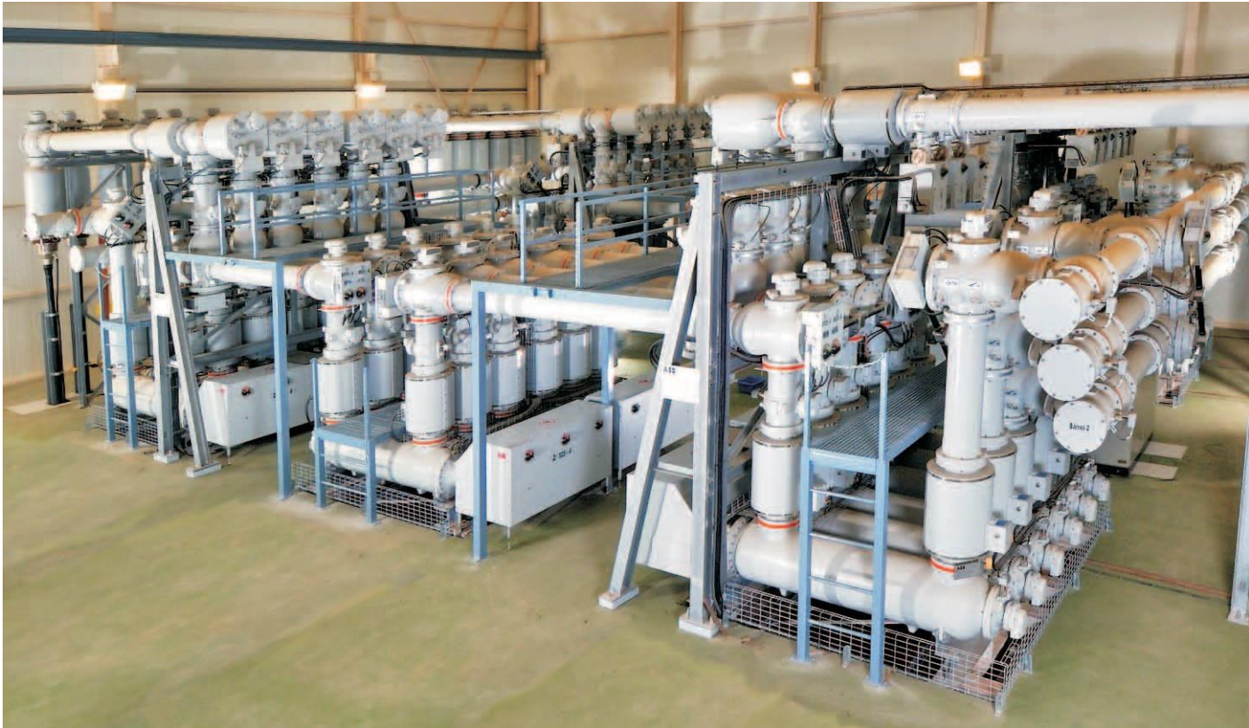
ELK-14 switchgear in 1½-breaker arrangement
