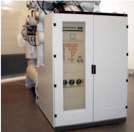
Local control cubicles
