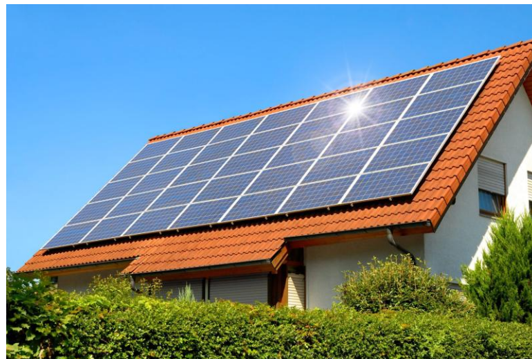
Figure 1: Example of a residential photovoltaic solar system.
