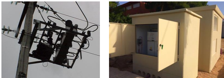
Figure 125: Right: Recloser; Left: Secondary substation (Iberdrola)
