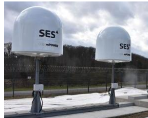
Figure 92: Parabolic antenna (SES)
