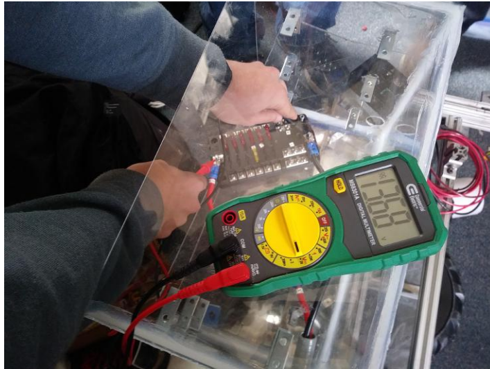
Image 34: Battery, Fuse Box and Thermal Breaker test
