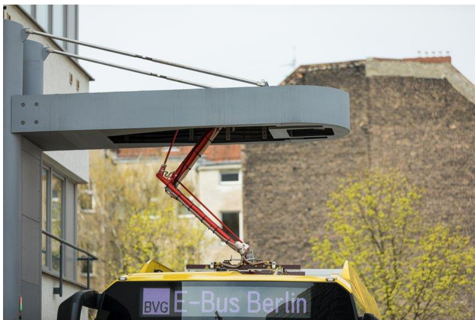
Figure 15: Innovative quick charging station for electric buses.
