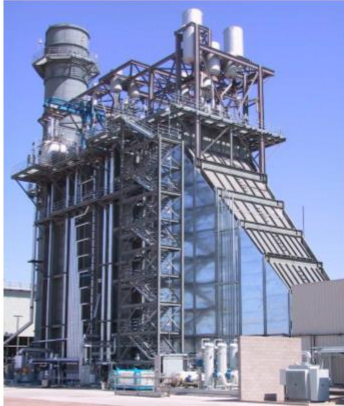
Figure 21- Heat Recovery Boiler, Source [Unión Fenosa Generación]
