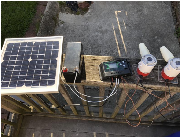
Figure (52). Solar circuit outside of the platform.
