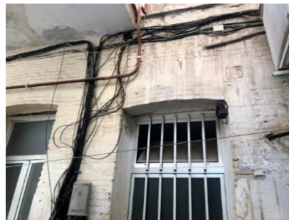
Figure 1. Deteriorated construction materials and unsafe electrical connections.
