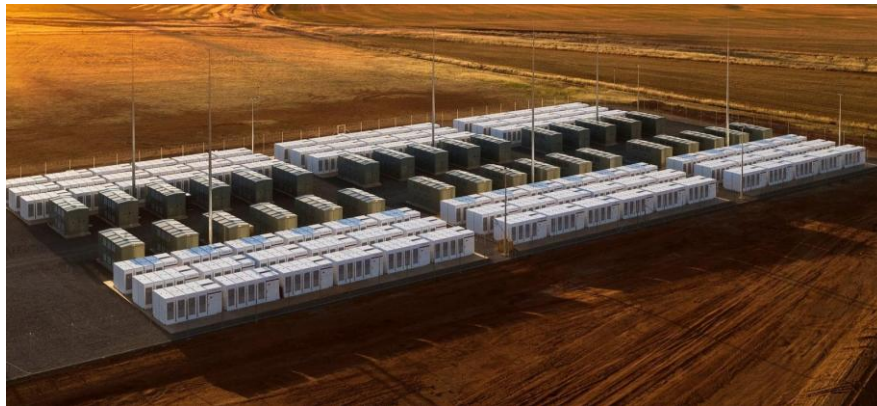
Figura 11. Proyecto BESS Hornsedale Power Reserve [Hornsedale]
