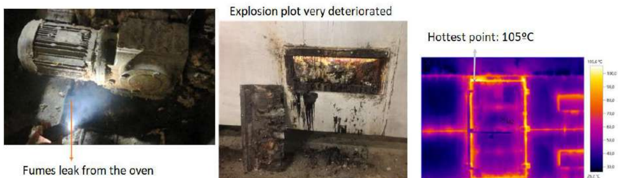
Figure 6: Elements deteriorated with leaks and with temperatures above their admissible range.
