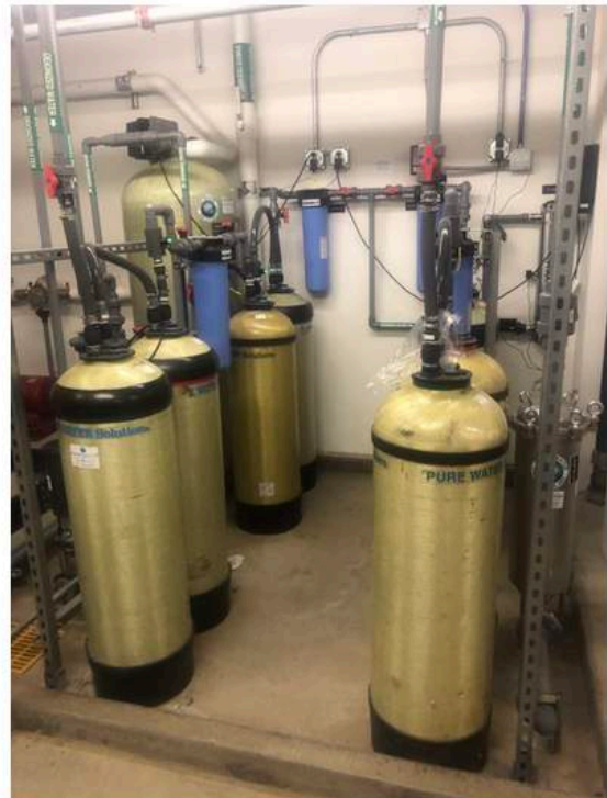
Figure 10: Pure water tanks
