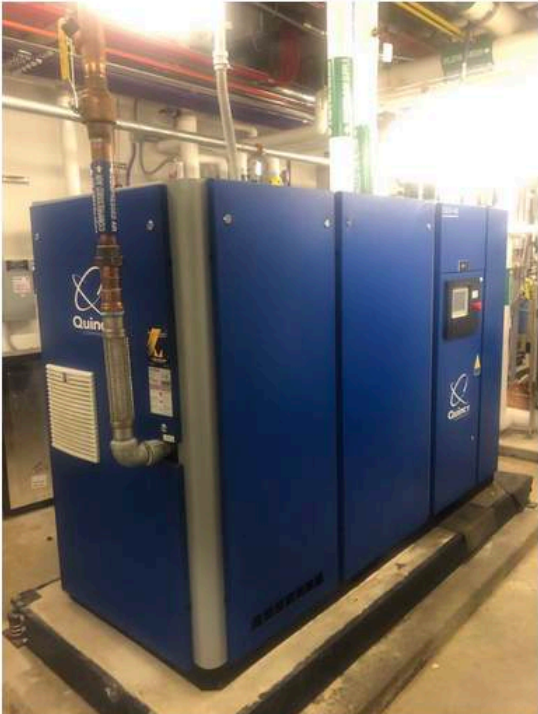
Figure 3: Primal air compressor
