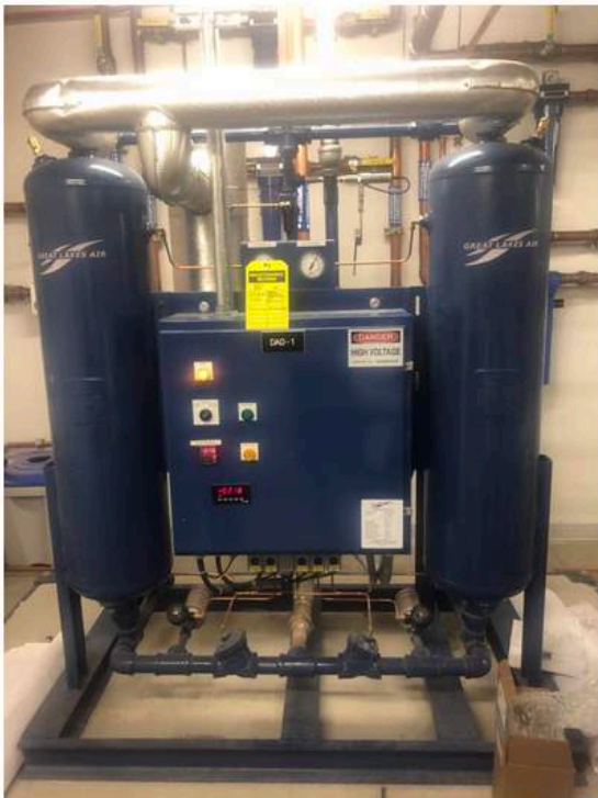
Figure 9: Compressed air system
