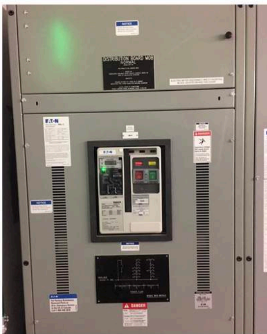
Figure 14: Main Distribution Board "MDB"
