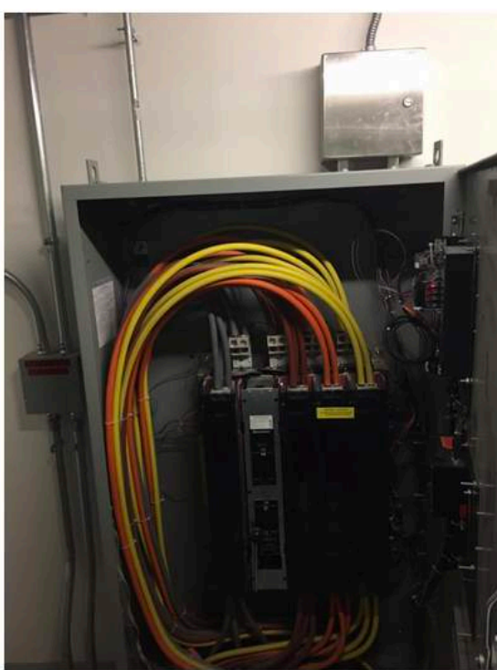
Figure 16: Wiring connection of switching unit
