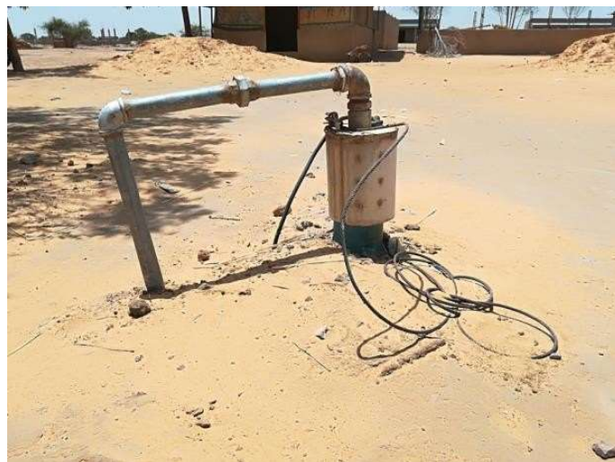
Illustration 4. Well with an electric pump out of service
