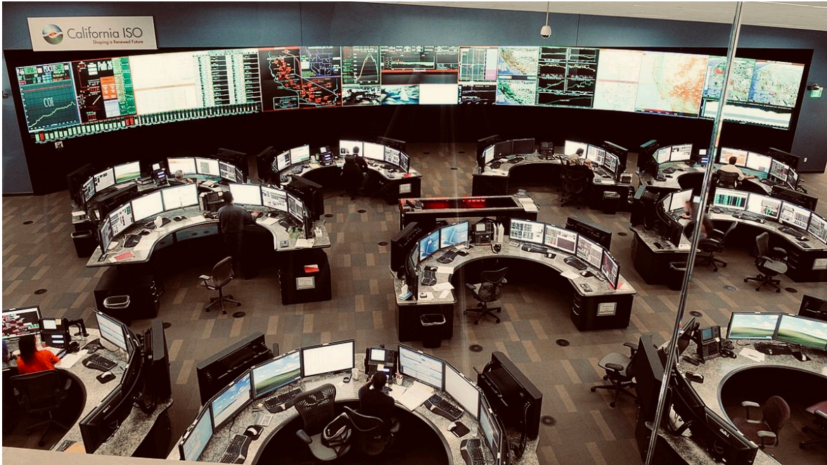
Figure 3: The control room at the California Independent System Operator headquarters in Folsom
