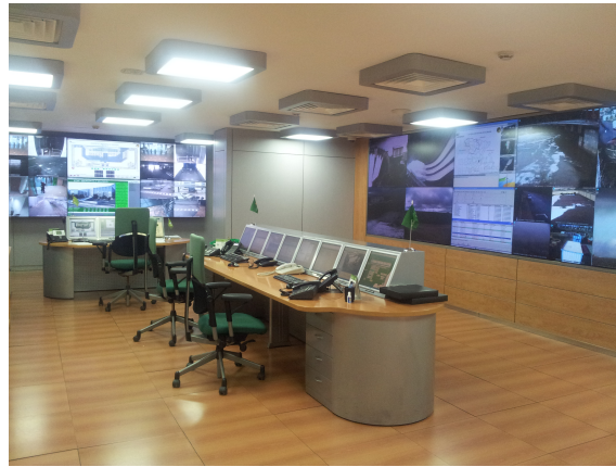
Figure 1.1. Example of a surveillance control center.
