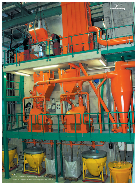
Figure 7.3: KEZO metal recovery facility [ZAR11]
