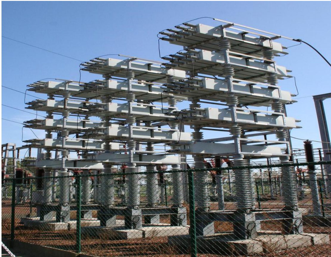
Figure 1- Capacitors being used to correct the power factor in industries
