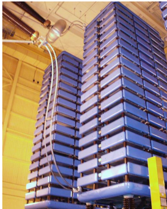
Figure 20. Thyristors Stack (Manitoba Hydro-Bipole)
