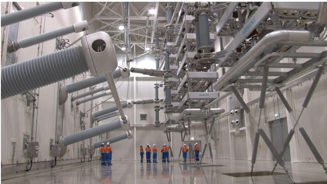
Figure 7. Thyristor Valves Hall
