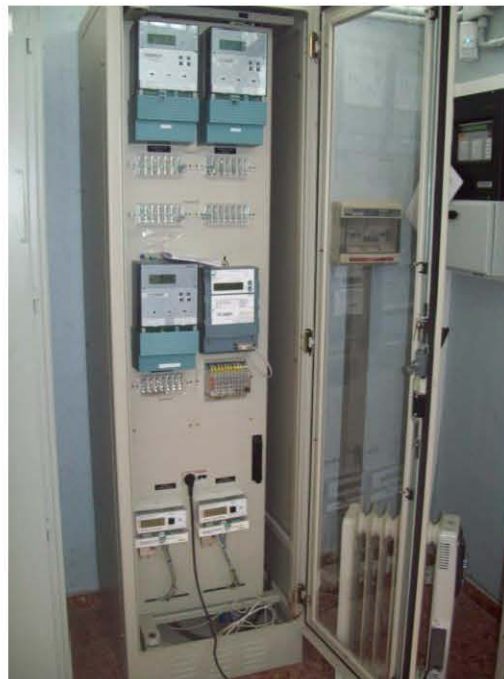
Figure 3-5. Figure of the metering equipment of a mini-hydro
