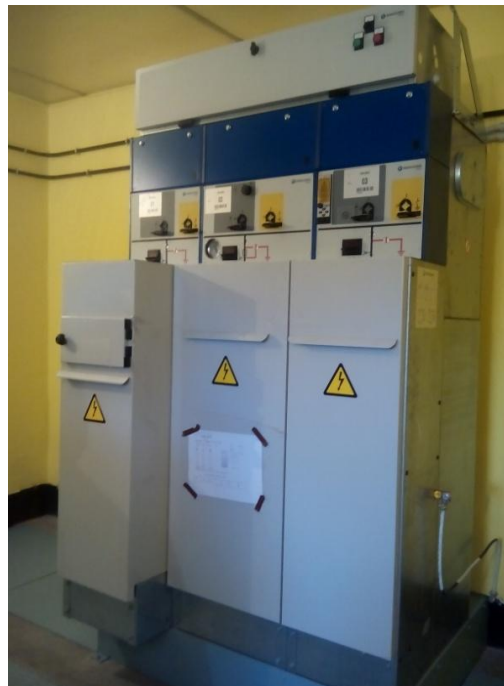
Figure 35. Cells of 28CBE5 Secondary Substation. Source: Own elaboration.
