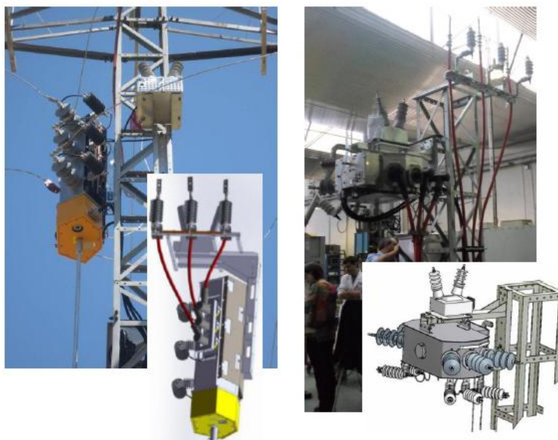
Figure 20. Switch-sectionaliser. Souce: Gas Natural Fenosa.
