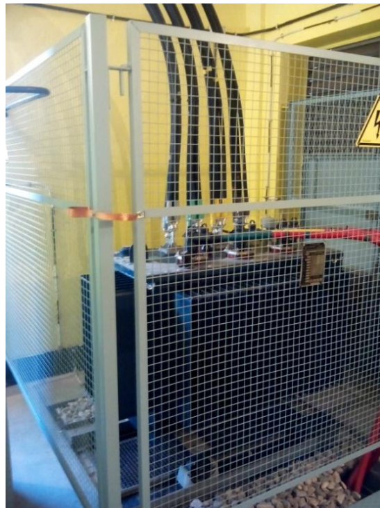
Figure 37. Transformer. Source: Own elaboration.
