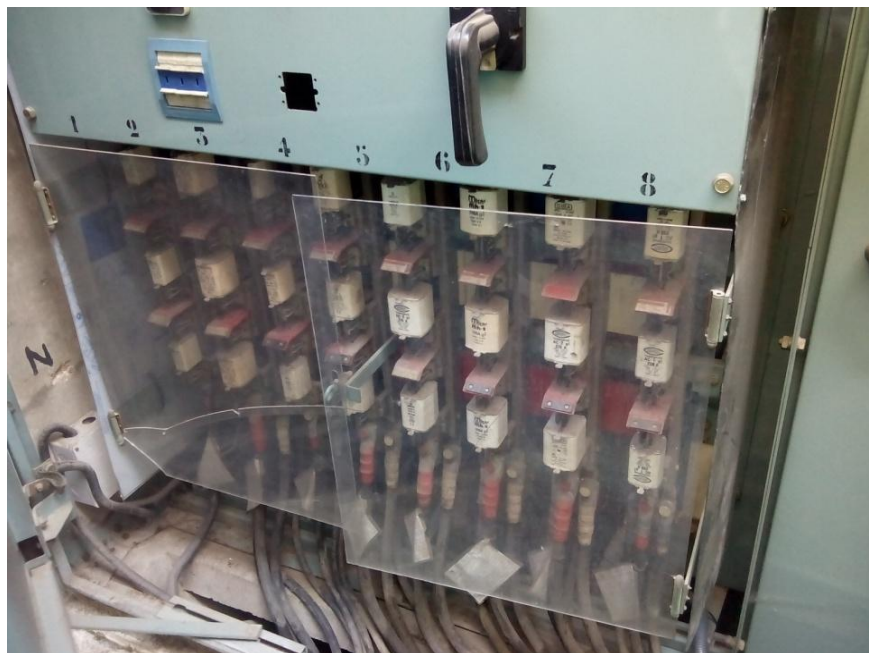
Figure 42. Output lines/feeders. Source: Own elaboration.
