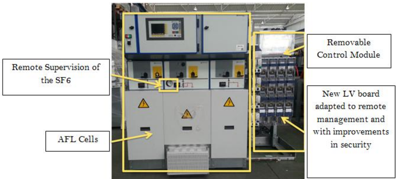
Figure 19. Improvements in security in a Secondary Substation. Source: Gas Natural Fenosa.
