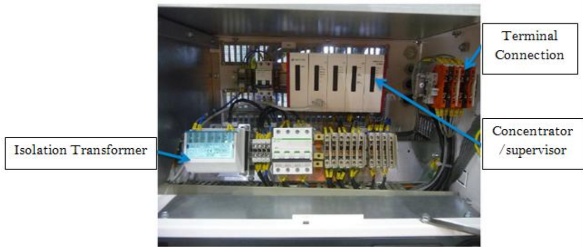
Figure 18. Remote management technology in a Secondary Substation (MV-LV). Source: Gas Natural Fenosa.
