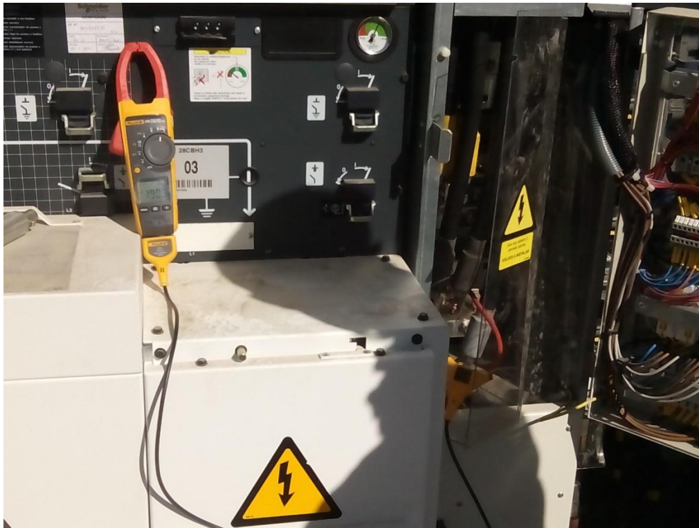
Figure 33. Metering of currents with Clamp. Source: Own elaboration.
