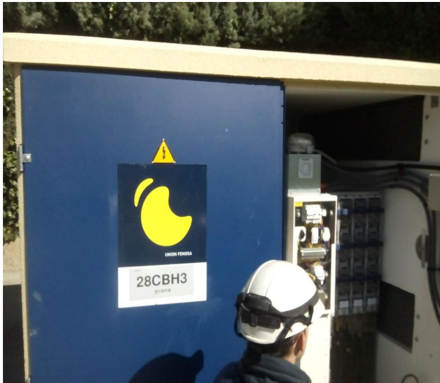
Figure 30. Outside and inside of SS 28CBH3. Source: Own elaboration.
