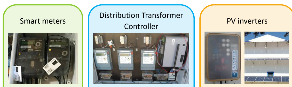
Figure 4-2 Pictures of the devices used in a centralised voltage control functionality (SUSTAINABLE project, 2016a)
