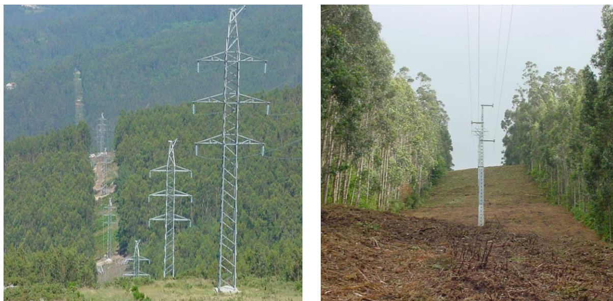
Figure 1-2 Facilities belonging to Gas Natural Fenosa
