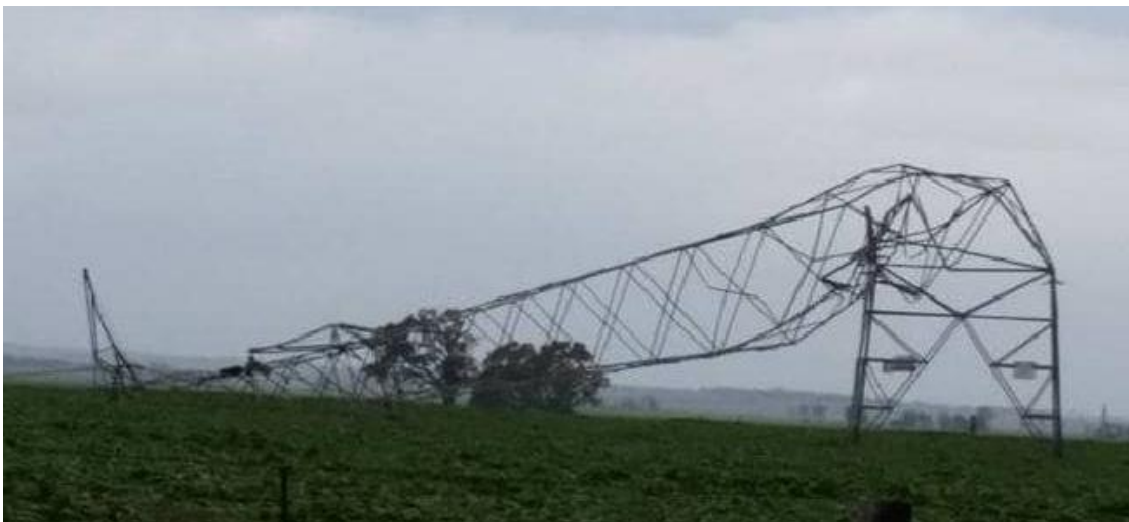
Figure 1 – Fallen electricity transmission tower after a storm in South Australia. Source: [8]
