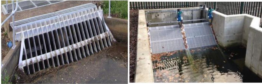
Figure 42. Left: Trash Rack, Right: Hydraulic Screen
