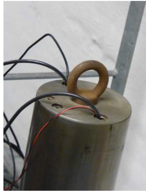
(b) Four cables going into the chamber.
