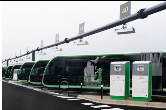
Figure 32. Irizar ie tram and Jema charging system
