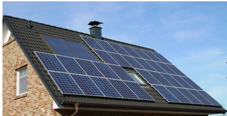
Figure 13. Coplanar rooftop installation
