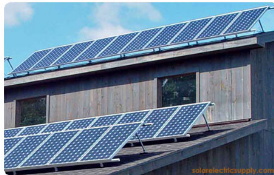
Figure 14. Sloped roof installations
