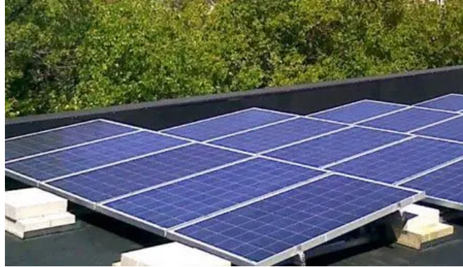
Figure 15. Flat roof installations
