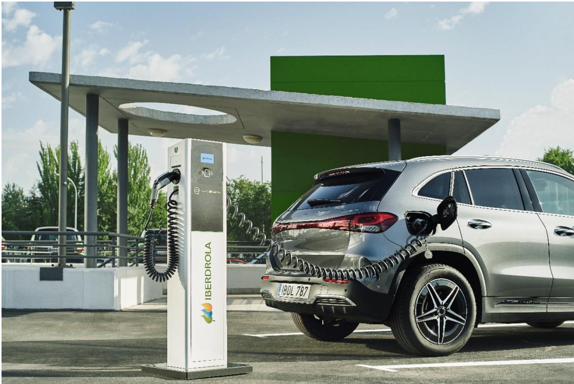
Figure 10: Charging point of an electric vehicle
