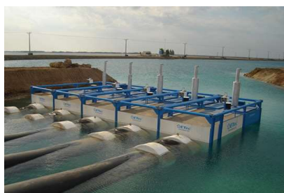
Figure 23. Filter-pump system (ETEC).
