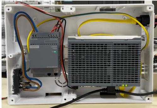
FIGURE 24. Gateway setup. The box includes power supply connectors that mitigate the risk of electrocution, along with Ethernet ports that allow direct connectivity to the case. This eliminates the need for threading RJ-45 connectors into the gateway ports, ensuring a simplified and efficient setup. Additionally, flexible USB connectors are incorporated to facilitate easy access to the ports of the device.
